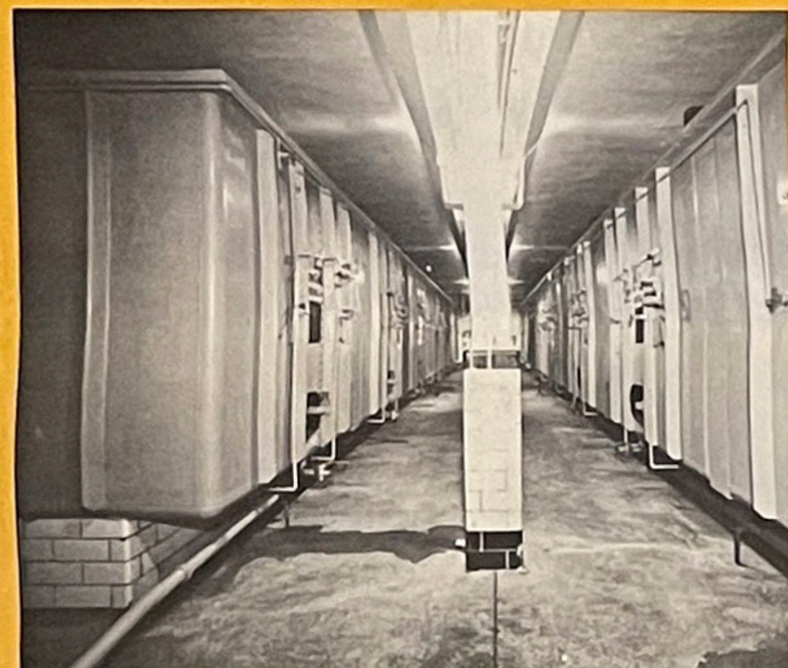
310 BBL. LASTIGLASS LINED STEEL RECTANGULAR OPEN FERMENTING TANKS
